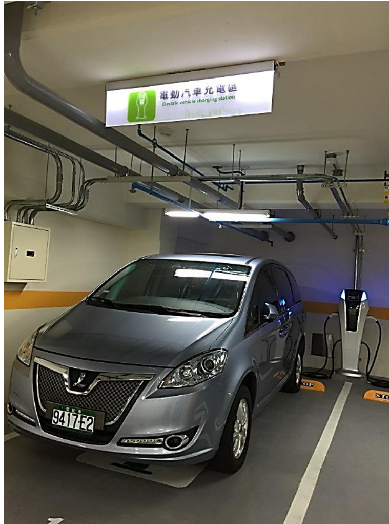
EV Charging Station
