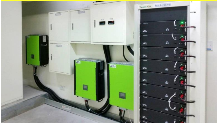
Energy storage systems in the Basement
