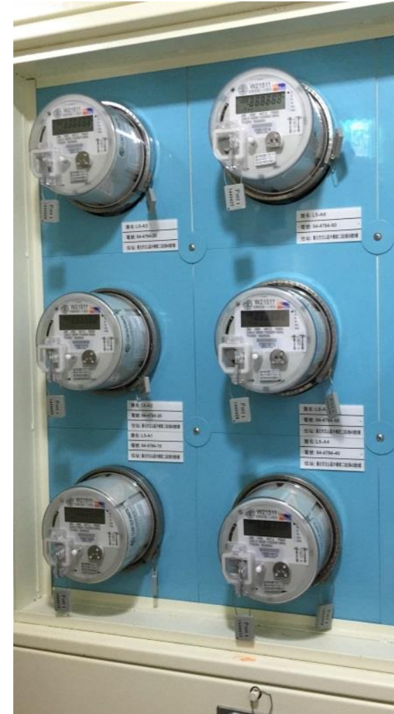
AMI- Smart Grid Infrastructure
